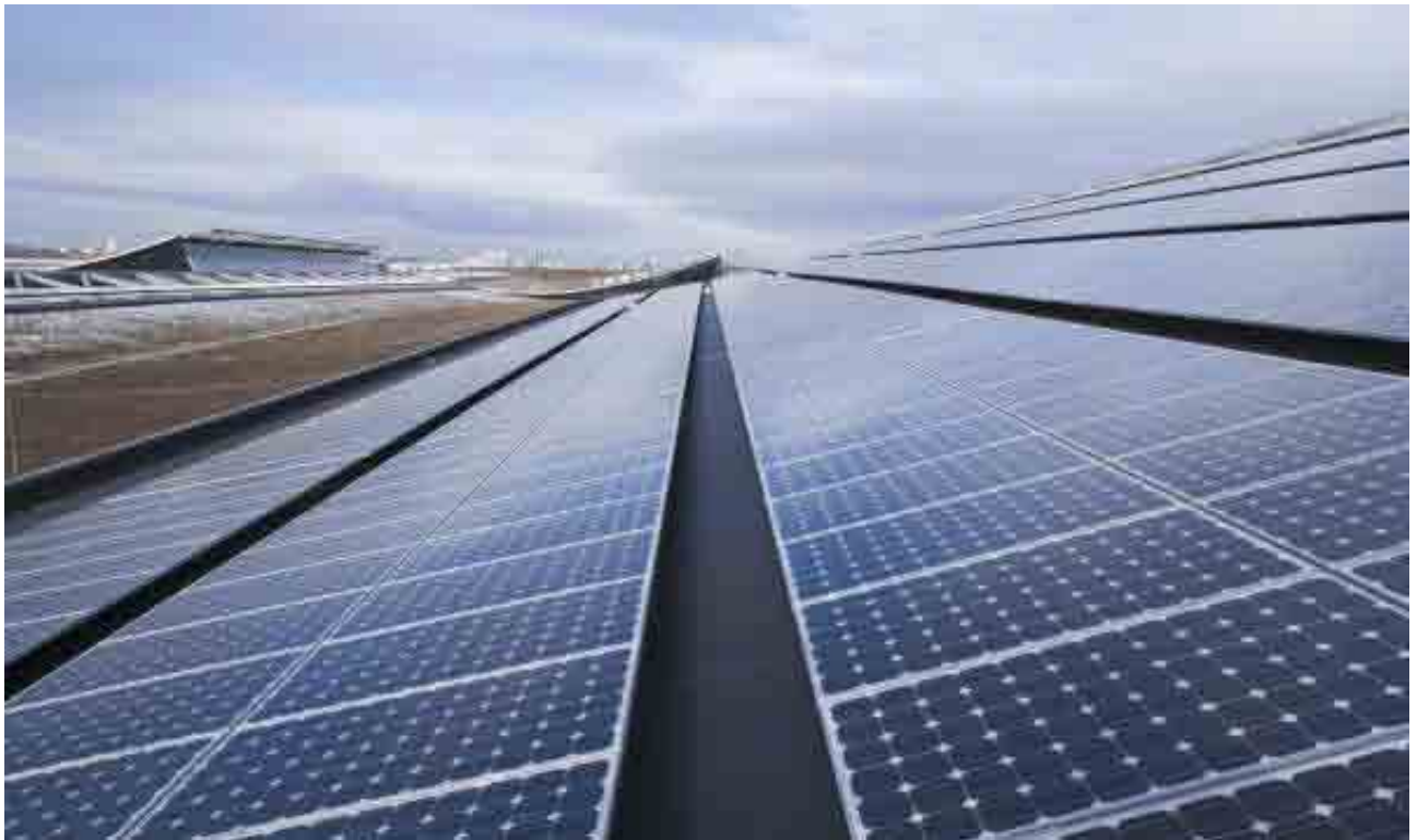
Stuttgart's new Trade Fair Centre: one of the world's largest photovoltaic roof systems.
